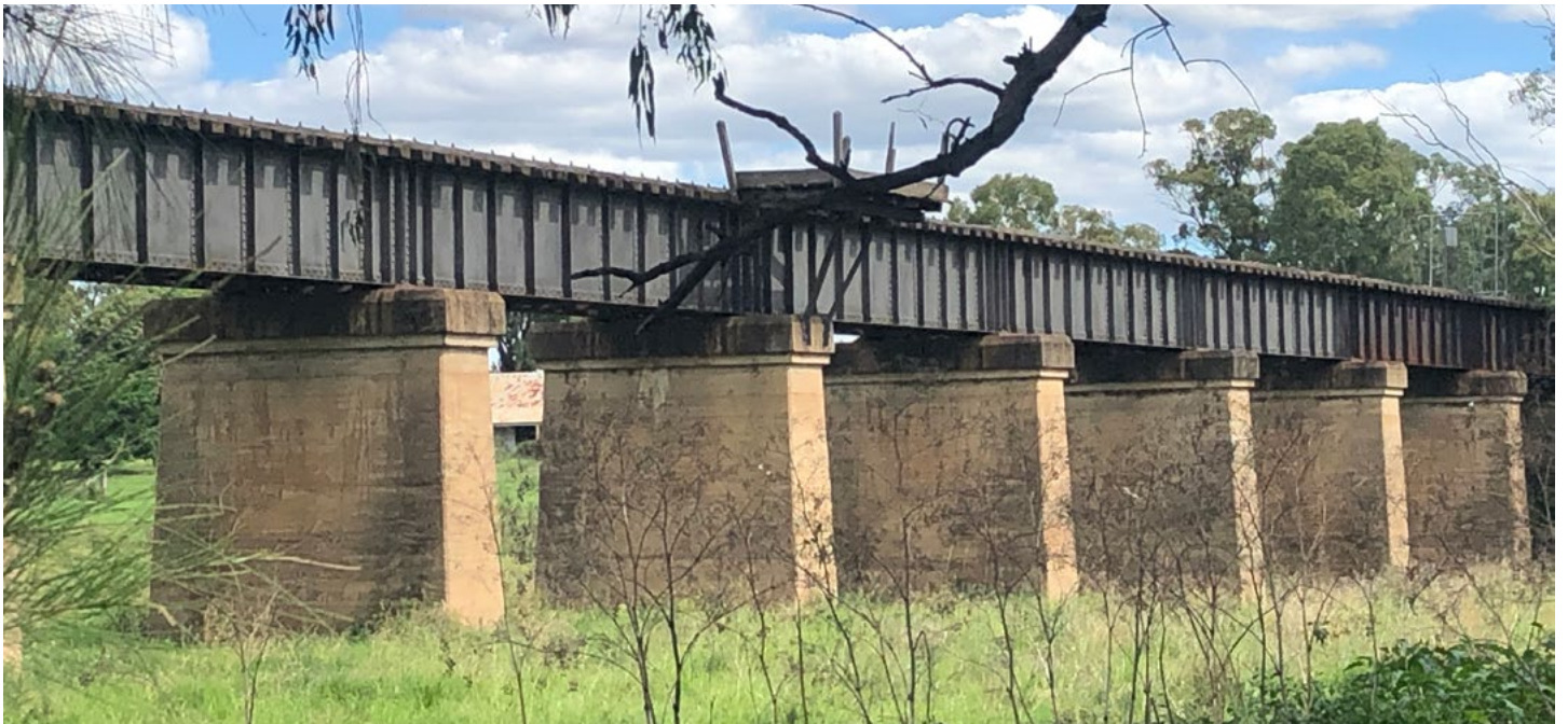
A section of the Dubbo-Toongi railway line spanning the Macquarie River floodplain.
