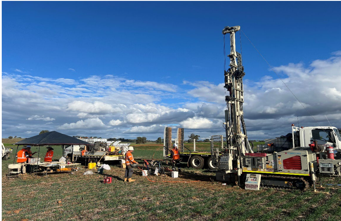
Geotech sampling to inform Front End Engineering Design – Dubbo Project Site . Photo taken 1 May 2024
