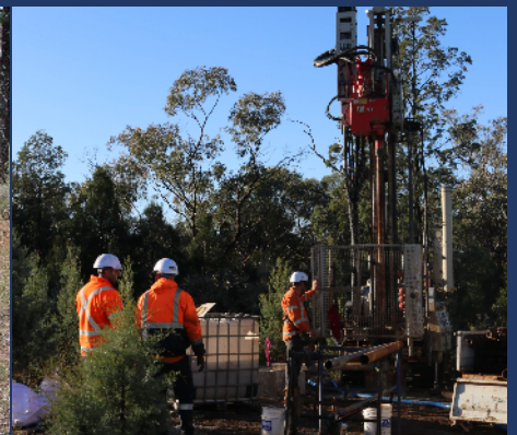
Core drilling and sampling work conducted as part of the REOA activities.
